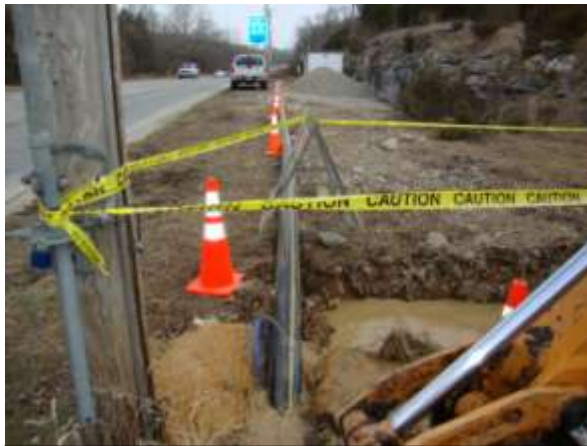
The construction of a natural gas line in Branson has started along Roark Valley Road.
